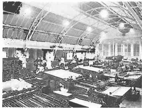
General Illumination of Press-Room with high candle-power Mazdalux units suspended close to the ceiling.
